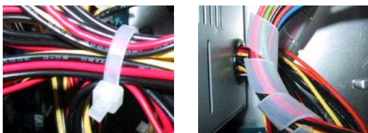
Fig. 7. Examples of bundling cords and cables
